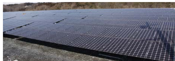
Ryoden Corporation Kurihara Power Plant (Miyagi Prefecture)
