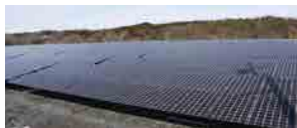
Ryoden Corporation Kurihara Power Plant (Miyagi Prefecture)
