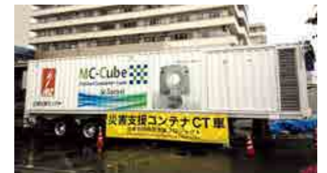
CT examination car with a container-shaped diesel generator: Kumamoto City Hospital (emergency aid provided in the aftermath of the Kumamoto Earthquake)
